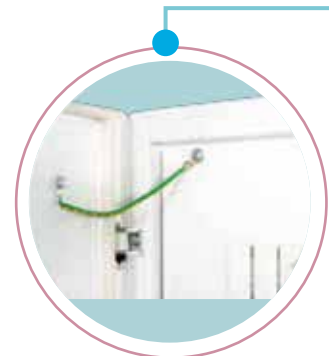
Door earthing in Enclosure for human safety
